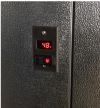
At an inspection, the temperature of this walk-in cooler was 48° which is too high to keep food safe. (The temperature should be 41° or lower.) The health inspector worked with the venue staff to quickly cool the food using other methods and to bring the walk-in temperature down to 41° before the food became unsafe to serve.
